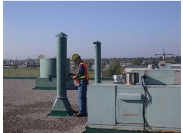
Depending on the site wind conditions, building geometry, and stack parameters, emissions from chemical fume hoods released through stacks may find their way back into the building at fresh air intakes.
