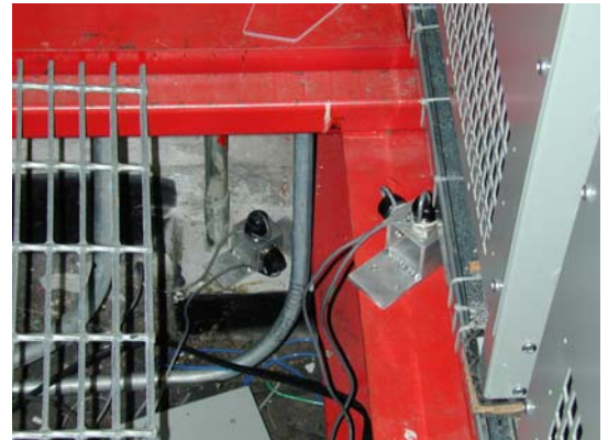
Using accelerometers to monitor and control vibrations from a mechanical penthouse
